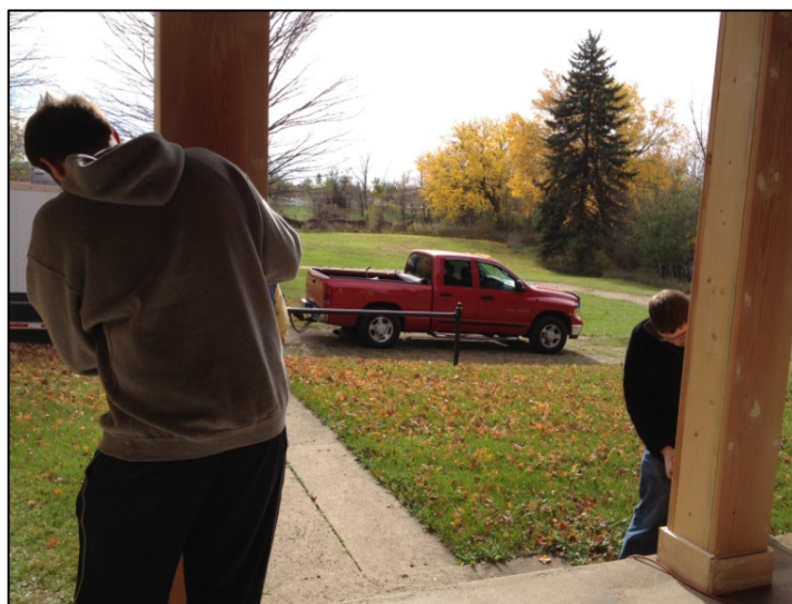
David Sellers and Jared Wabeke, sanding the pillars on the front porch. (Photo by Shino Toma)
